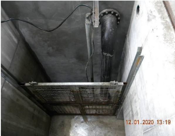
Figure 36 : View from above of the chamber with the pump. Picture 1
