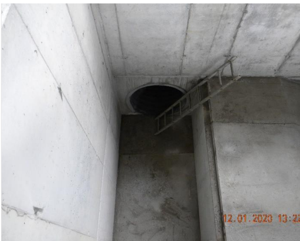
Figure 34 : view from above of the chamber with entry of the pipe. Picture 1
