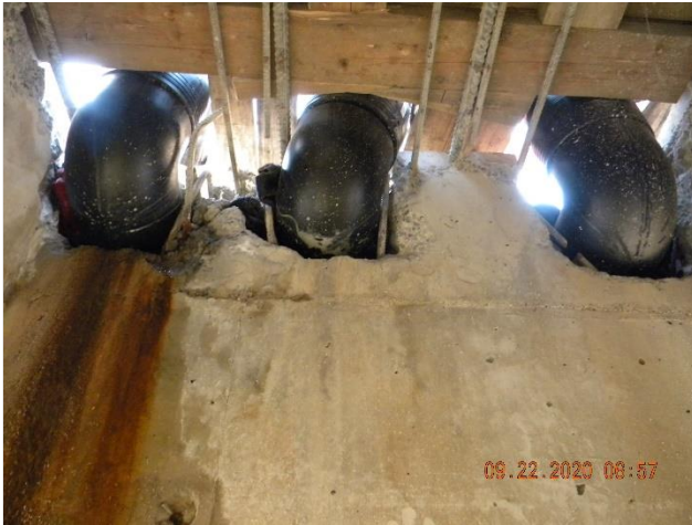
Figure 31 : View of drainage pipes for dewatering pumps
