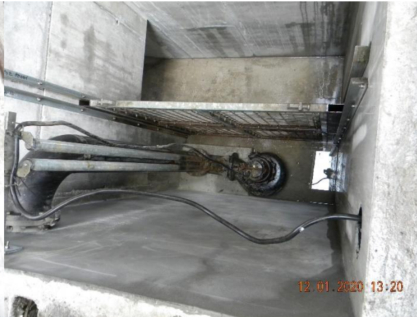
Figure 37 : View from above of the chamber with the pump. Picture 2
