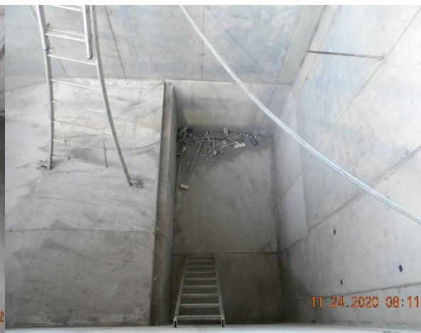
Figure 35 : view from above of the chamber with entry of the pipe. Picture 2
