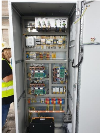
Figure 2 : The electrical cabinet
