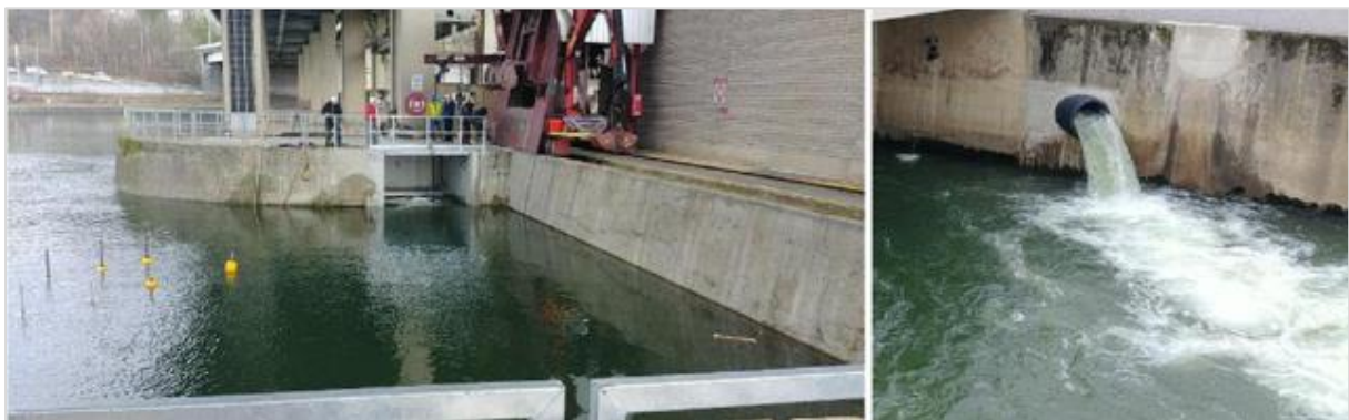
Figure III-7: Entrance and exit of the outlet set up for the passage of salmon smolts
