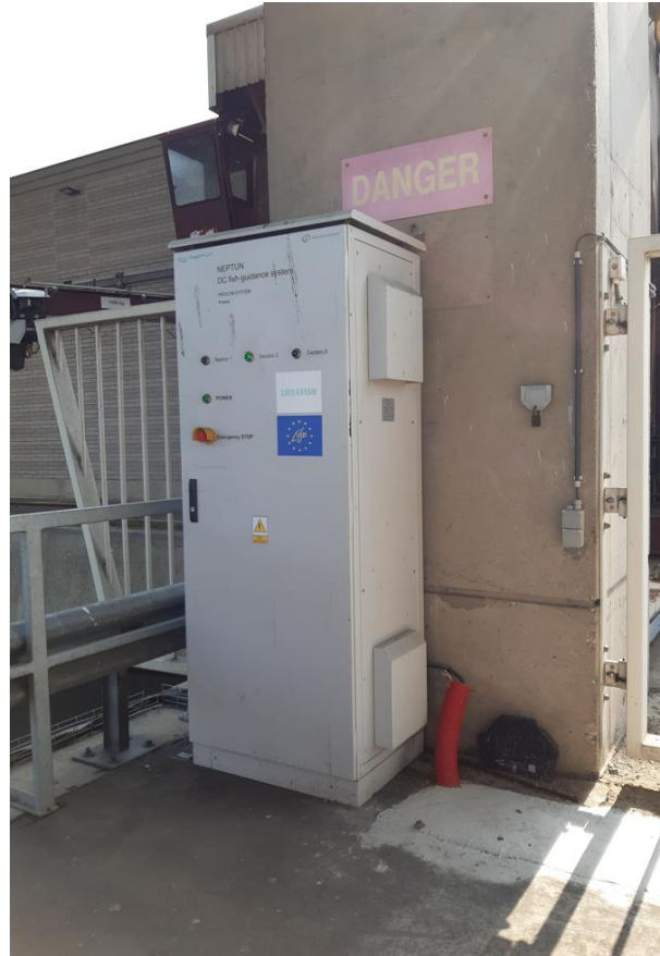
Figure IV-21: Illustration of the electrical box installed at the Grands-Malades power plant
