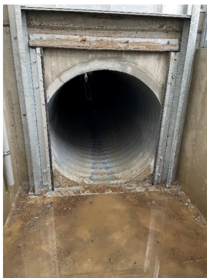
Valve at the outlet entrance
