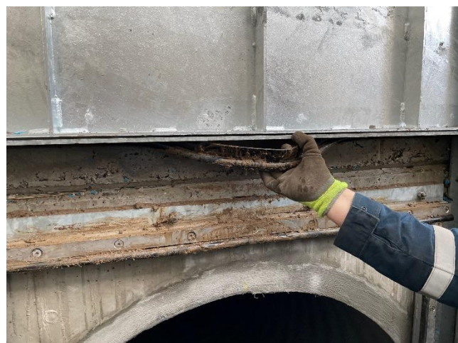
Valve gasket is not positioned correctly view 1
