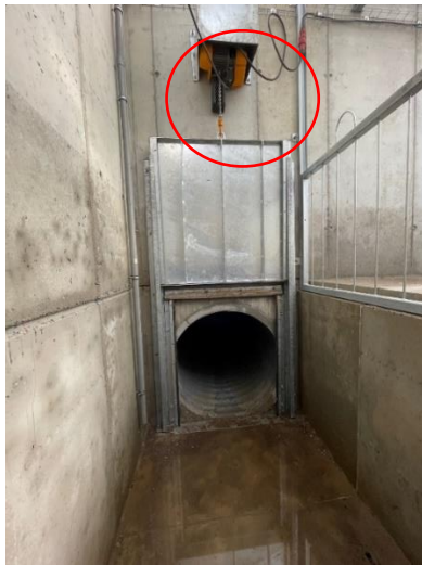
Hoist of the valve
