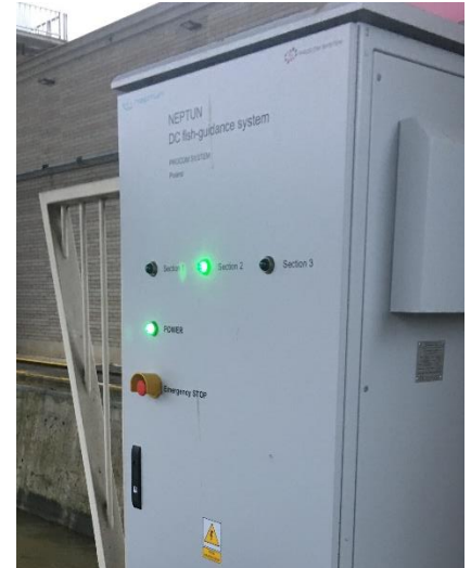
Error on the electrical cabinet
