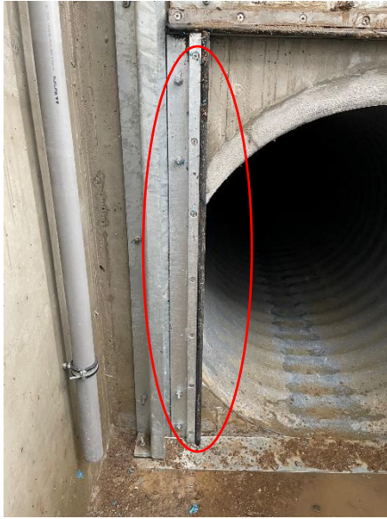
Valve gasket is not positioned correctly view 2
