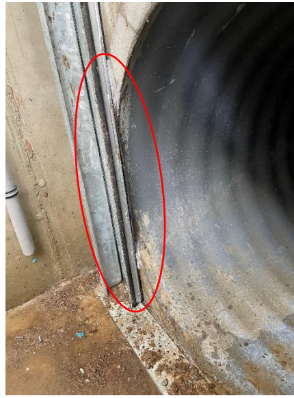
Valve gasket is not positioned correctly view 3
